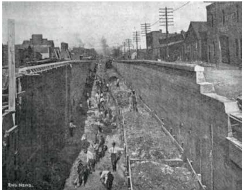
Looking East from 22nd Street After Core Excavation, Showing Work of Dressing Roadbed.
